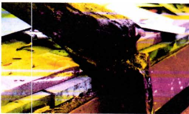
The endgrain of the topsides frame is sometimes only slightly affected by rot. If only a small section can be cut from the topsides frame, the shape of the bottom frame can be adjusted to compensate.
