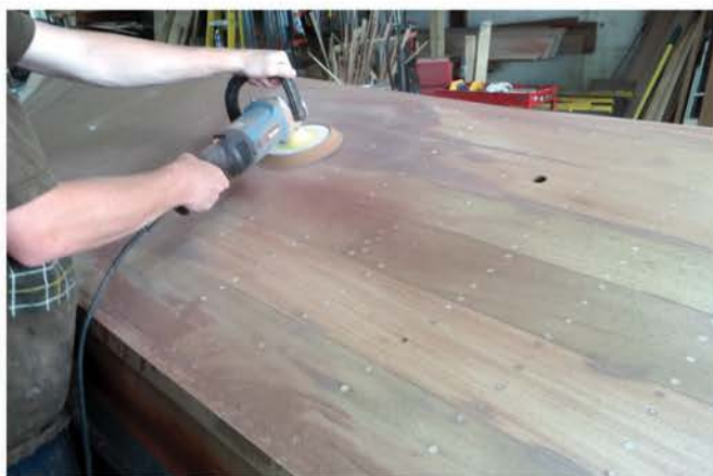
Complete removal of incorrect paint coatings to allow applications of CPES, barrier coat primer, and bottom paint.
