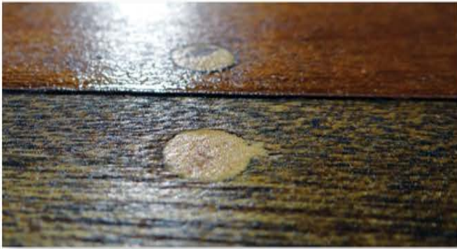
Some tiny gaps are too small to force 5200 into. Three quarts of CPES caused the wood to swell, then set in that condition. Note the raised rubber.
